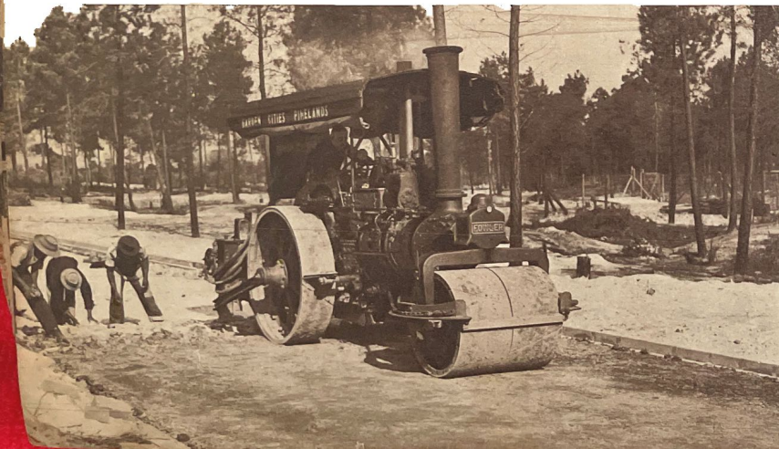
Garden Cities has its own roadmaking machinery at Pinelands and lays out streets ahead of the building of houses.
